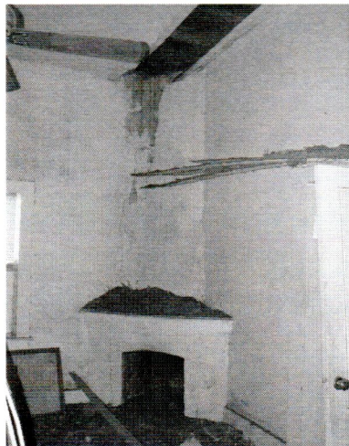
Original corner fireplace showing ceiling collapse due to a roof leak.
